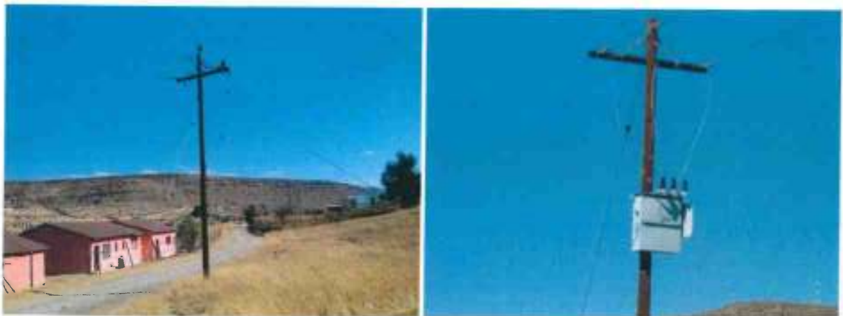
Photo 9: Electricity supply at Thembeni site
